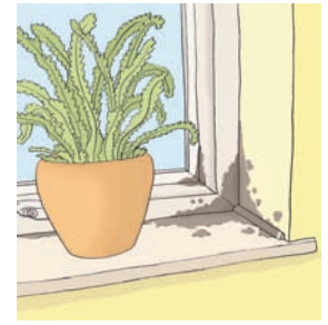
mould and damp
